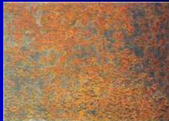
Rust Grade B
