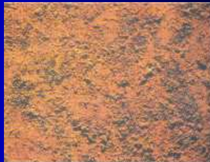
Rust Grade D
