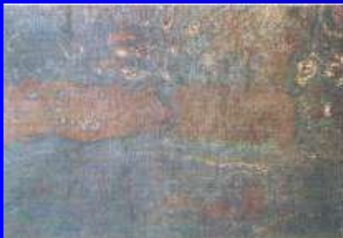
Rust Grade A
