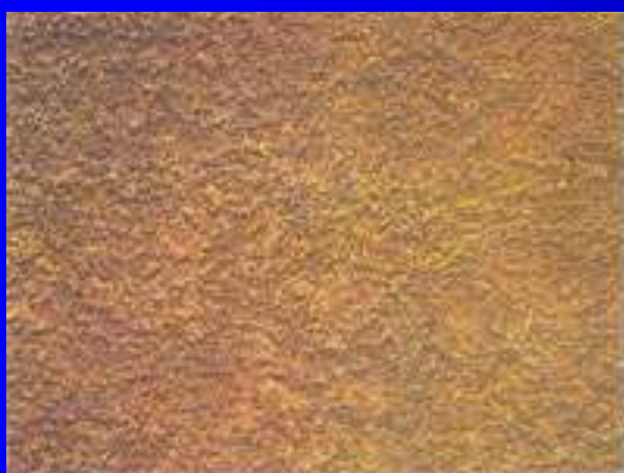
Rust Grade C
